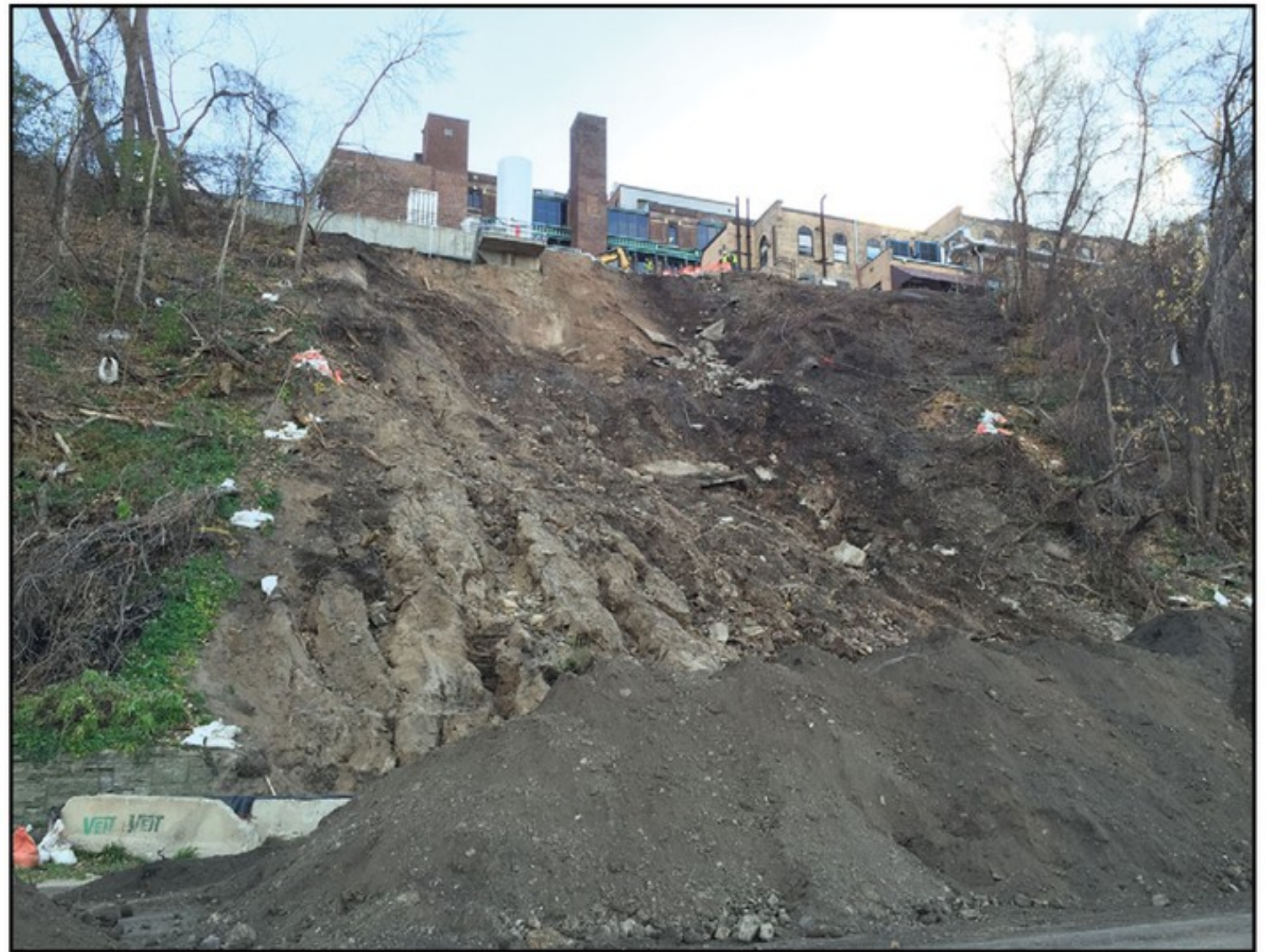
4,000 cubic yards of soil was dislodged on June 19th of 2014 after 4.2 inches of rain fell on already saturated ground.
