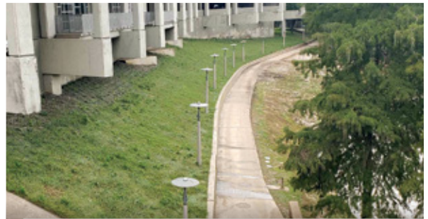
When flood waters receded, the slope remained intact—proving the green solution was a viable one.
