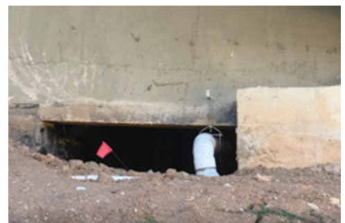
Strong currents from Hurricane Harvey compromised the base of the Bayou Place complex, flooding the building and shutting those facilities down.
